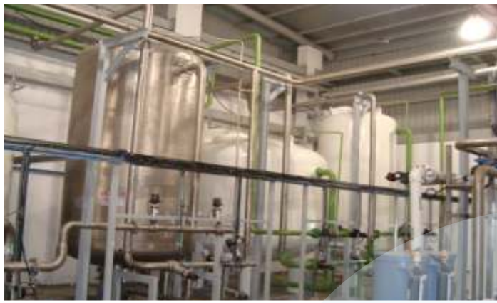
Pressure Sand & Activated Carbon Filters
